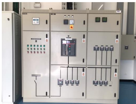
Main Distribution Board (MDB) 400 V
